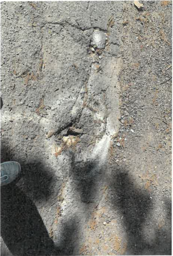
locations that backed up water has found its way to the surface. Water runs down the hill and ends up in the resident's crawlspace
