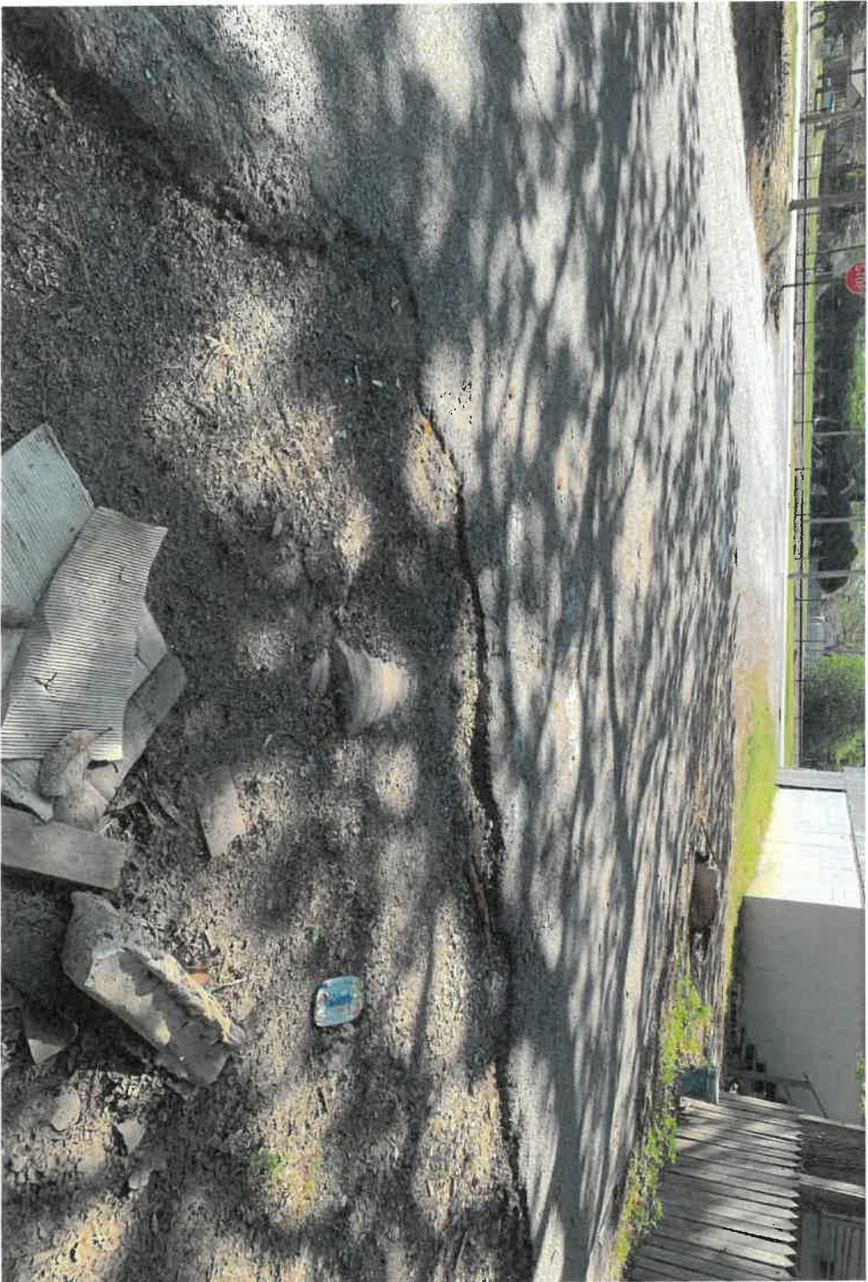
Exposed pipe along W 19th Street
