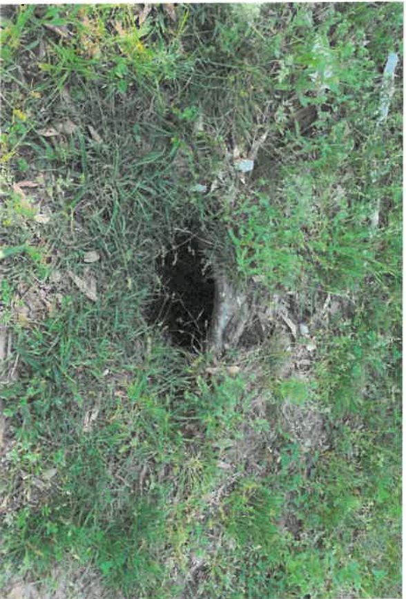
Exposed pipe at Willow Street
