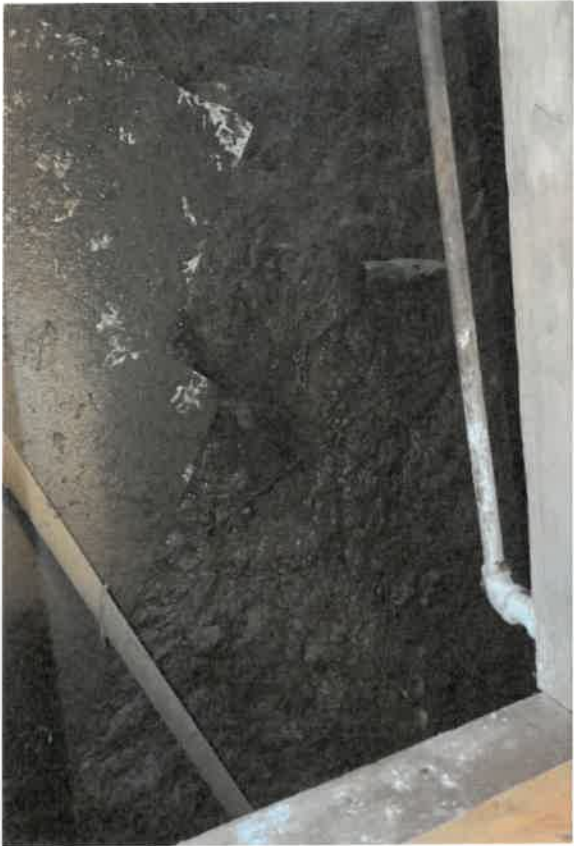
water in residents crawlspace after 2 weeks of no rain
