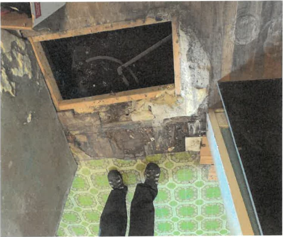
water damage above the southwest corner of the house
