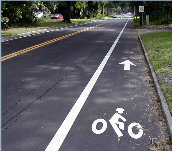
Bold striping and markings remind drivers that bicyclists belong on the road
